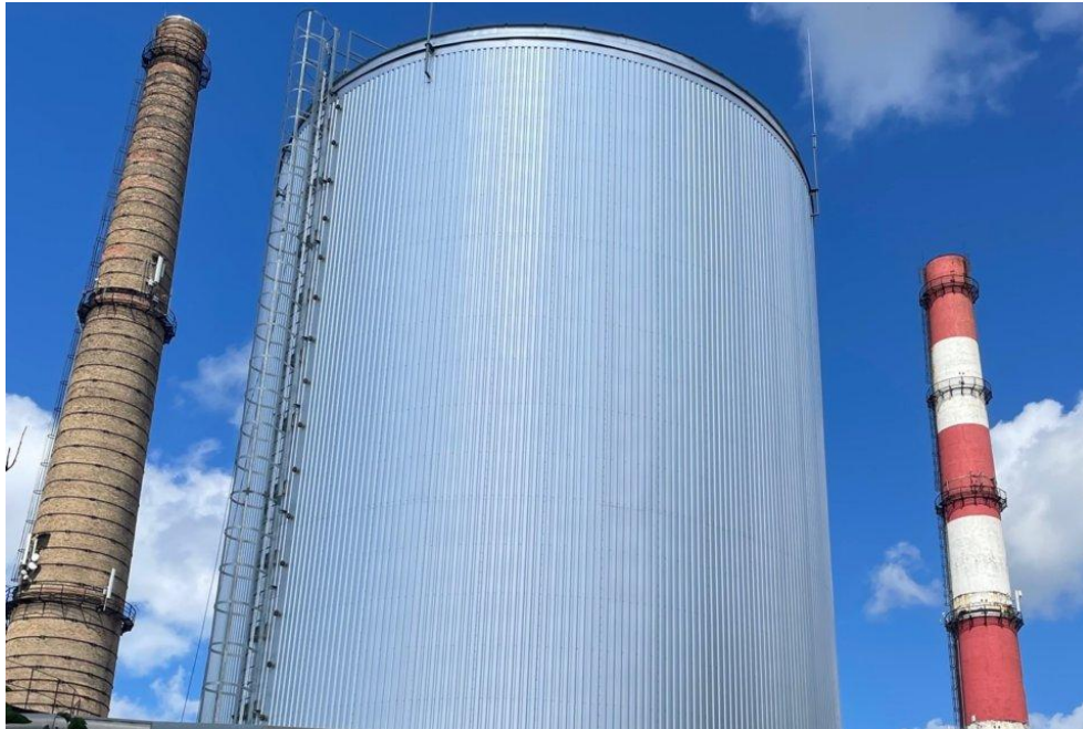
Fig. 4. The heat storage in Klaipėda City (Photo by Klaipėda Energy)
